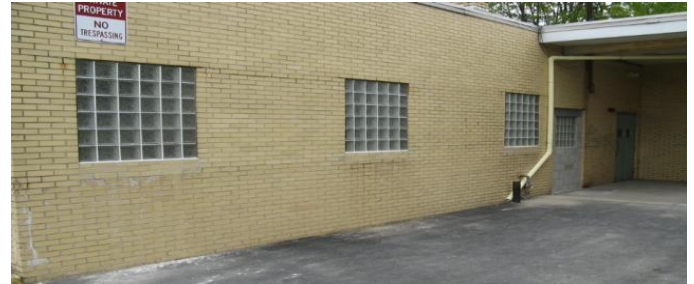
The new glass block windows and glass block/concrete block replacement for the mechanical room door. (Photo by Frank Warner)
