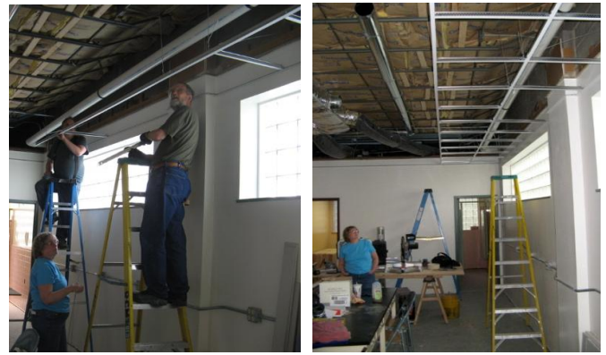
(Left) Ellen and Don Schwarzkopf and Frank Warner begin installation of the ceiling grid in the jewelry room. (Right) Ellen inspects the initial two rows of grid. (Photos by Frank Warner)
