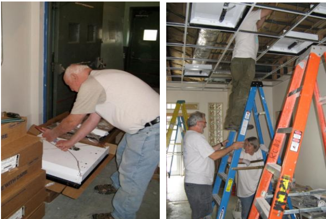
(Left) Merrill Dickinson prepares light fixtures for installation. (Right) John Chickadel, Lola Fields, and Joe Pizzirusso install light fixtures in the central classroom. (Photos by Frank Warner)
