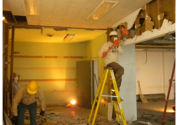
Lola Fields, Roger Binns, and Doug Wiggins continue the demolition process. (Photo by Drew Schmith)
