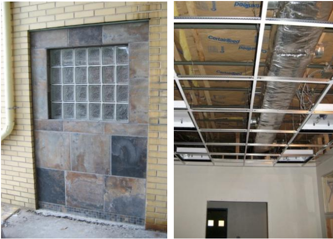
(Left) Finished tile and glass block in the former mechanical room exterior door opening. (Right) Ceiling grid installation is complete and lights have been placed in the grid. (Photos by Frank Warner)
