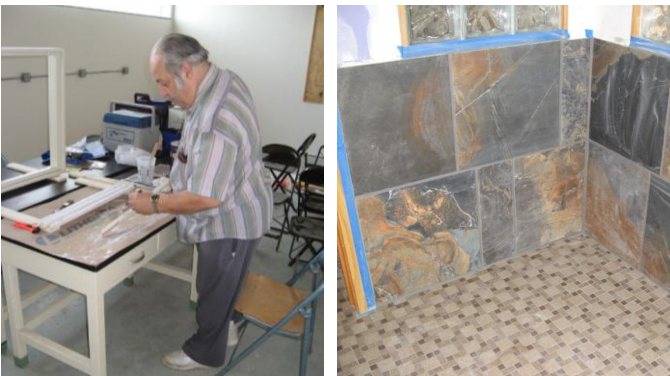
(Left) Pete Santucci paints window frames. (Right) Doug Klieger (not shown) adds grout to the tile in the vestibule. (Photos by Frank Warner)
