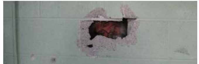
Don Schwarzkopf breaks through the cinder block wall, the beginning of a new interior door into the mechanical room. (Photos by Frank Warner)
