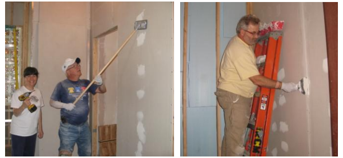
(Left) Sue Manuel and Bill Mattis work on drywall. (Right) John Chickadel applies tape and mud to drywall joints. (Photos by Frank Warner)
