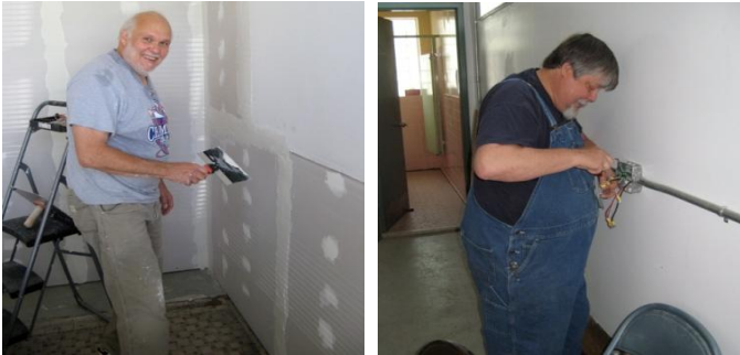
(Top) Bill Mattis (left) cuts insulation while Joe Pizzirusso (right) installs drywall. (Bottom) Jim Johnston (left) applies mud to drywall joints in the library and Don Schwarzkopf (right) wires an electrical receptacle.
