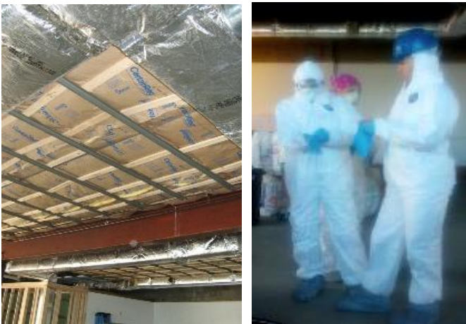
(Left) Rigid insulation is installed above the ceiling; each piece cut to fit. (Photo by Frank Warner) (Right) Karissa supplied special suits to protect the insulation installation crew from loose particles of fiberglass. (Photo by Lola Fields)
