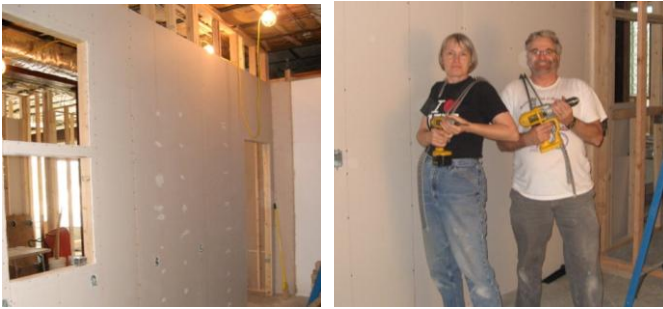
(Left) The drywall on one side of the jewelry room is completed. (Right) Lola Fields and John Chickadel pose as drywall bandoleers; on their shoulders are strips of drywall screws! (Photos by Frank Warner)
