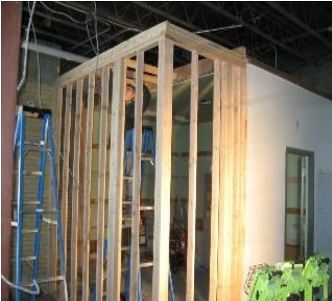
Lola Fields adds joists to complete storage room framing. (Photo by Frank Warner)
