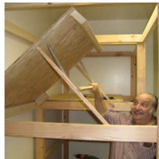
Pete Santucci demonstrates the lift scheme for the storage room shelving unit. (Photo by Frank Warner)
