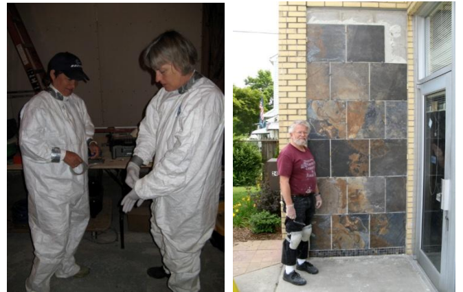
(Left) Charlotte Moore and Lola Fields 'suit up' for insulation installation. (Right) Doug Klieger installs tile at the entrance. (Photos by Frank Warner)
