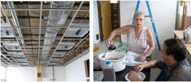
(Left) Lighting fixtures are added to the ceiling grid in the jewelry room. (Right) Margie Marshall serves lunch to Don Schwarzkopf and the rest of the work crew. (Photos by Frank Warner)
