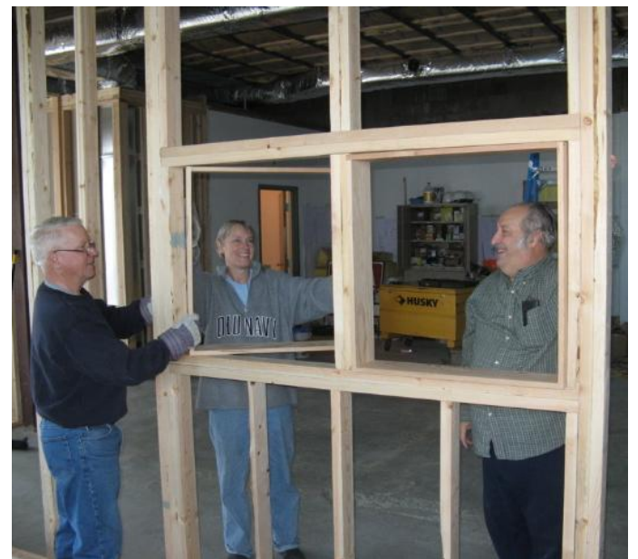
Bill Mattis, Lola Fields, and Pete Santucci admire their handiwork — a portion of a classroom wall with windows. (Photo by Frank Warner)
