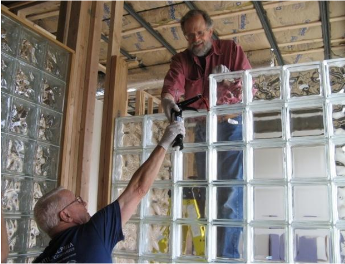
Bill Mattis and Frank Warner install a large interior glass block window. (Photo by Lola Fields)
