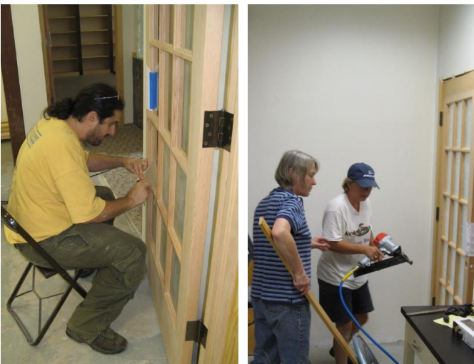
(Left) Joe Pizzirusso removes protective coating from door glass. (Right) Lola Fields and Charlotte Moore install door trim.
