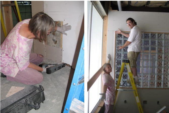
(Left) Lola Fields installs drywall. (Right) Lola and Joe Pizzirusso complete the drywall installation. (Photos by Frank Warner)
