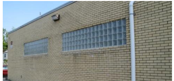
Glass block is installed to replace the windows on the side of the building.
