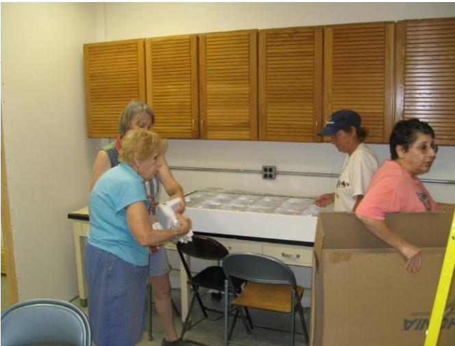
Lola Fields, Betty Margerum, Charlotte Moore, and Pam Wingrod prepare a lighting fixture for installation. (Photos by Frank Warner)
