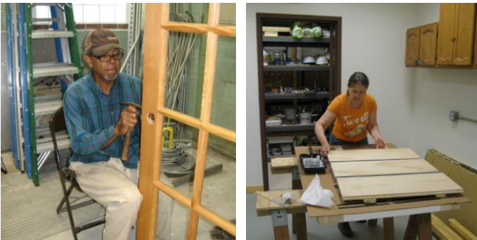
(Left) Doug Wiggins installs door hardware. (Right) Heidi Thompson paints Genie bench parts. (Photos by Frank Warner)
