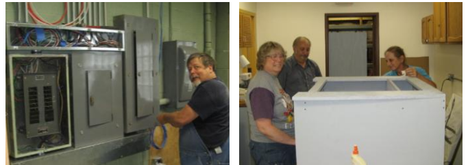
(Left) Don Schwarzkopf installs electrical panel covers in the mechanical room. (Right) Ellen Schwarzkopf, Pete Santucci, and Katy Winters assemble a Genie bench. (Photos by Frank Warner)
