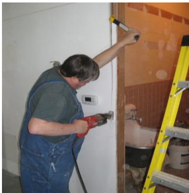
Don Schwarzkopf uses his Sawzall to remove old framing from the utility room door. (Photo by Frank Warner)
