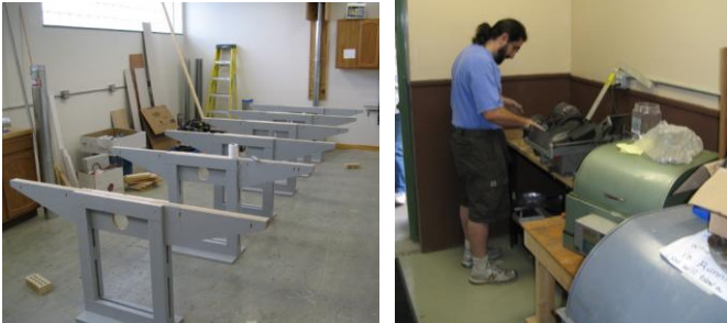
(Left) Supporting structures for the jewelry bench are laid out. (Right) Joe Pizzirusso installs trim saws. (Photos by Frank Warner)
