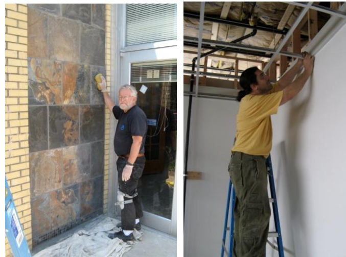
(Left) Doug Klieger grouts the large tile wall outside the front door. (Right) Joe Pizzirusso assembles part of the ceiling grid in the jewelry room. (Photos by Frank Warner)
