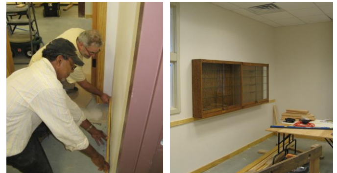
(Left) Doug Wiggins and John Chickadel install baseboards. (Right) Memorial Cases are installed in the central classroom.
