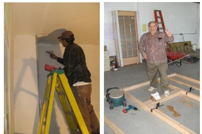
(Left) Doug Wiggins applies joint compound in the storage room. (Right) Pete Santucci works on the framing for the inner vestibule wall. (Photos by Frank Warner)
