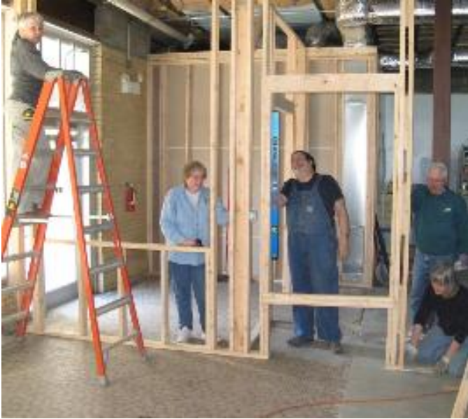
The framing crew, comprised of Karissa Hendershot, Ellen and Don Schwarzkopf, Bill Mattis, and Lola Fields, works on the wall separating the vestibule from the office. (Photo by Frank Warner)
