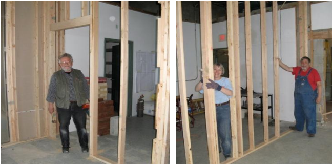
(Left) Doug Klieger with newly framed wall. (Right) Lola Fields and Don Schwarzkopf with the last section of the classroom wall.
